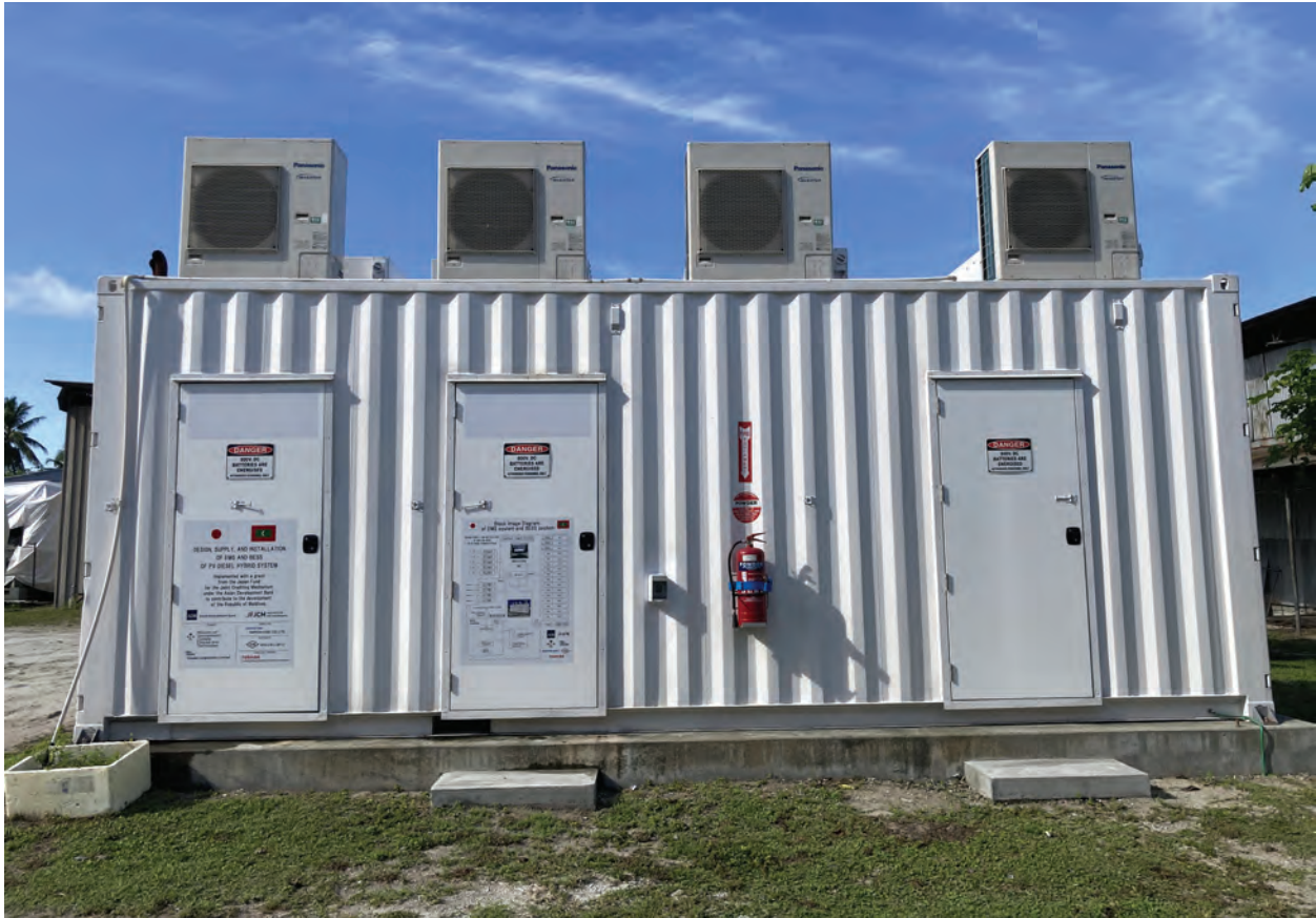
Advanced battery energy storage system installed in Addu City. Technologically advanced battery energy storage system was installed in Addu City (photo by Takahiro Murayama/ADB).
