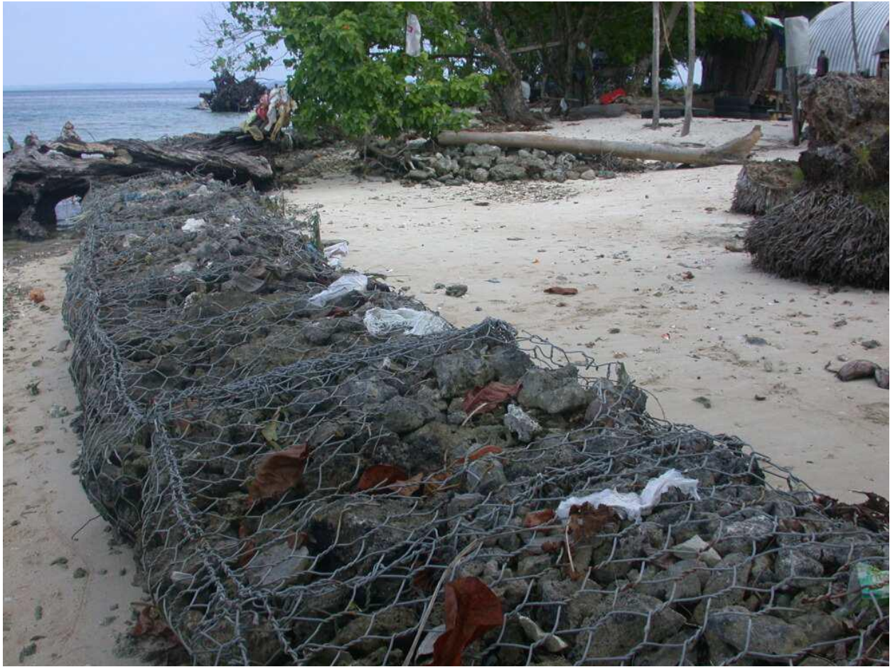
Figure 7: Gabion baskets used as modern coastal protection systems in the Los Negros Islands
