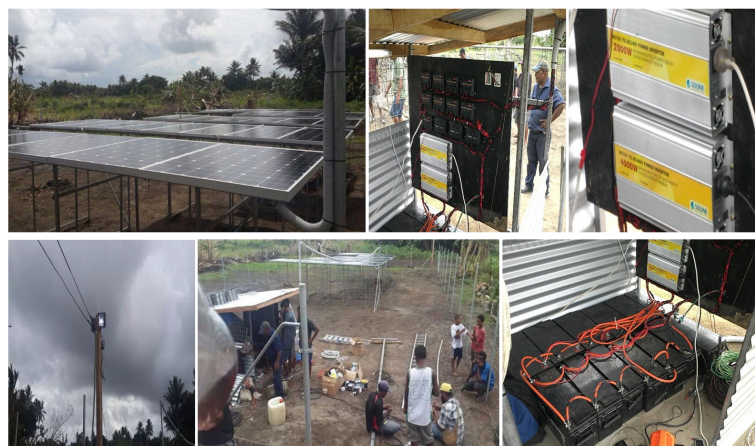
Paramana Village Community Solar Farm Project.
