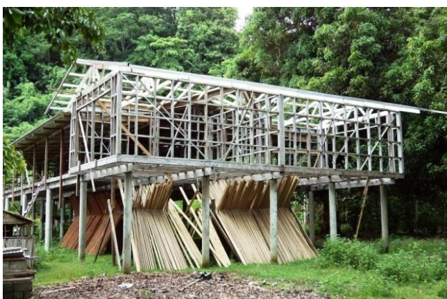
Figure 4: Primary school building under construction, a community supported own initiative (photo by P. Ramohia).
