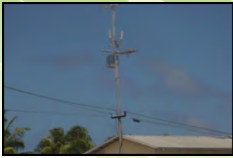
A Communication tower in Nauru powered by Solar Panels
