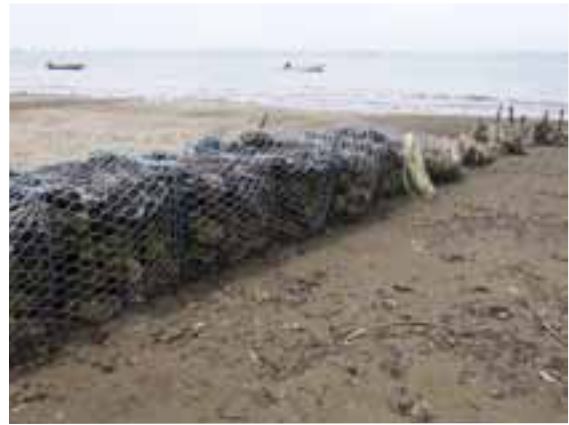
Plate 5. A local attempt to build a groyne to slow down rapid coastal erosion. This groyne made from gabion wire and rocks fell apart in less than two years. The other side of the groyne experienced rapid erosion after it was built.
