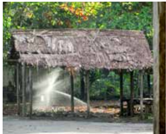
Plate 23. Water supply standpipe in need of repair
