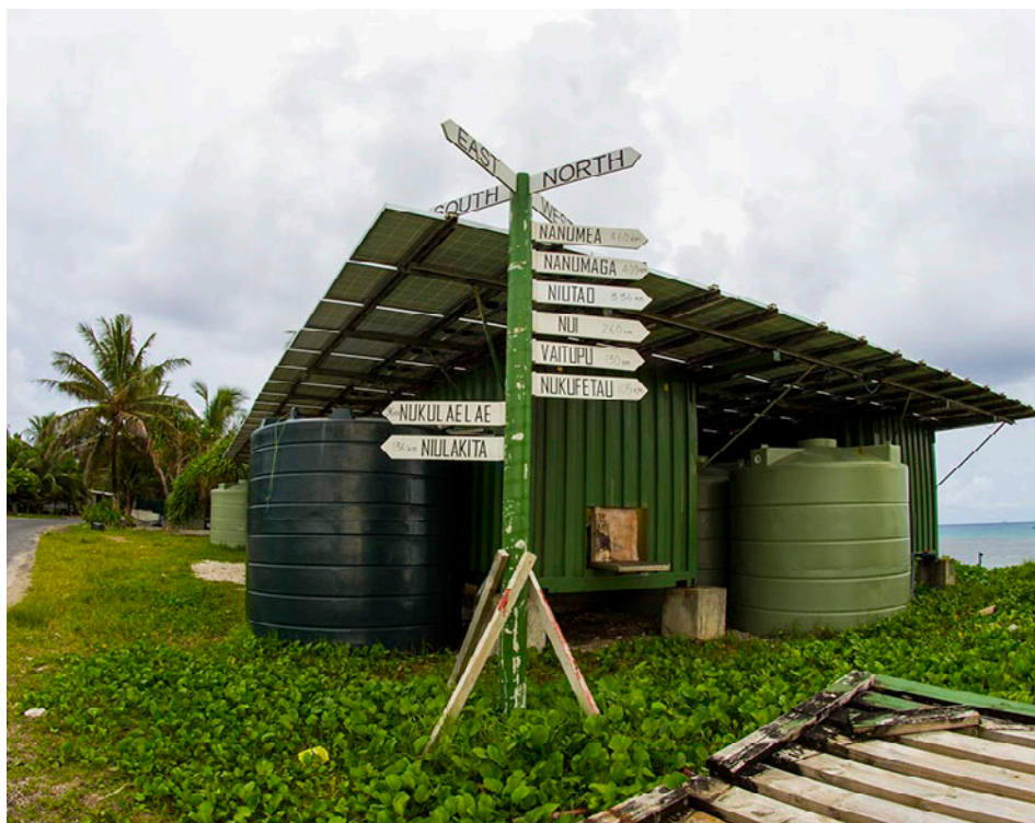
ABOVE: Desalination plants—like this solar-powered facility found on Funafuti—help offset the impacts of prolonged drought and saltwater intrusion on Tuvalu's fresh water supplies. Photo by C-CAP.
