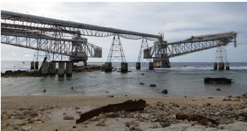
LEFT: Infrastructure for loading phosphate, the mining of which has resulted in the pollution of groundwater in Nauru. Photo by C-CAP.
